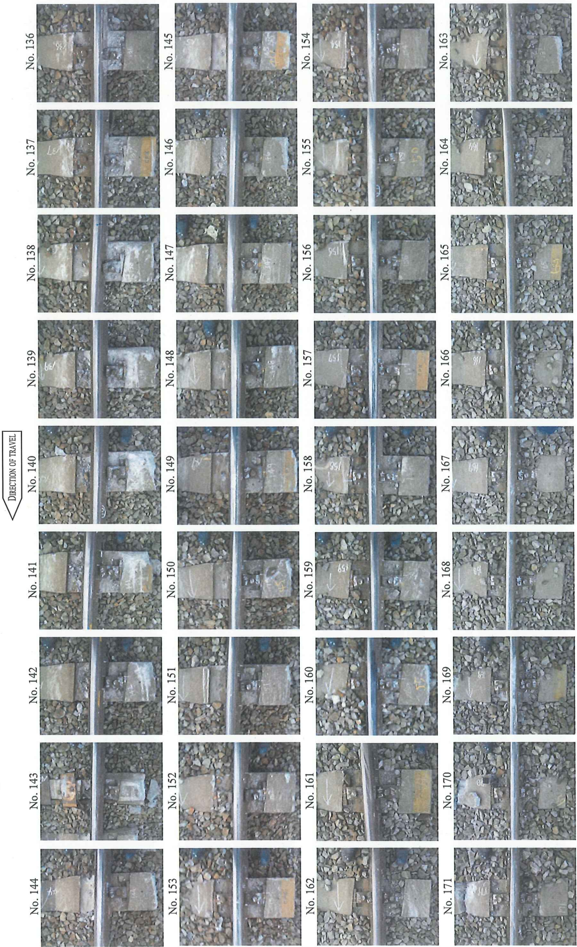
Figure 7 - States of Damage to Railway Facilities etc. (4) (Sleepers on the left rail side of the up track, 2/3)
