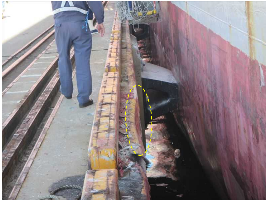
Figure 7 Damage to the quay
