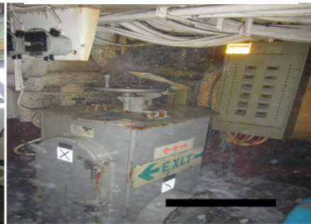
Inside damage ②
