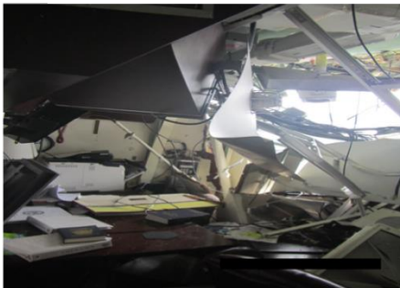
Inside damage ①
