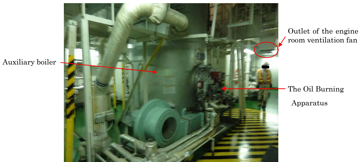
Photo 2.5-5 Outlet of the engine room ventilation fan at port side of the Oil Burning Apparatus
