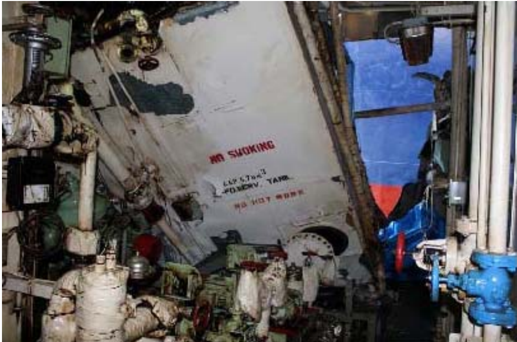
Photo 3: Damage to Ship A (Engine Room)
