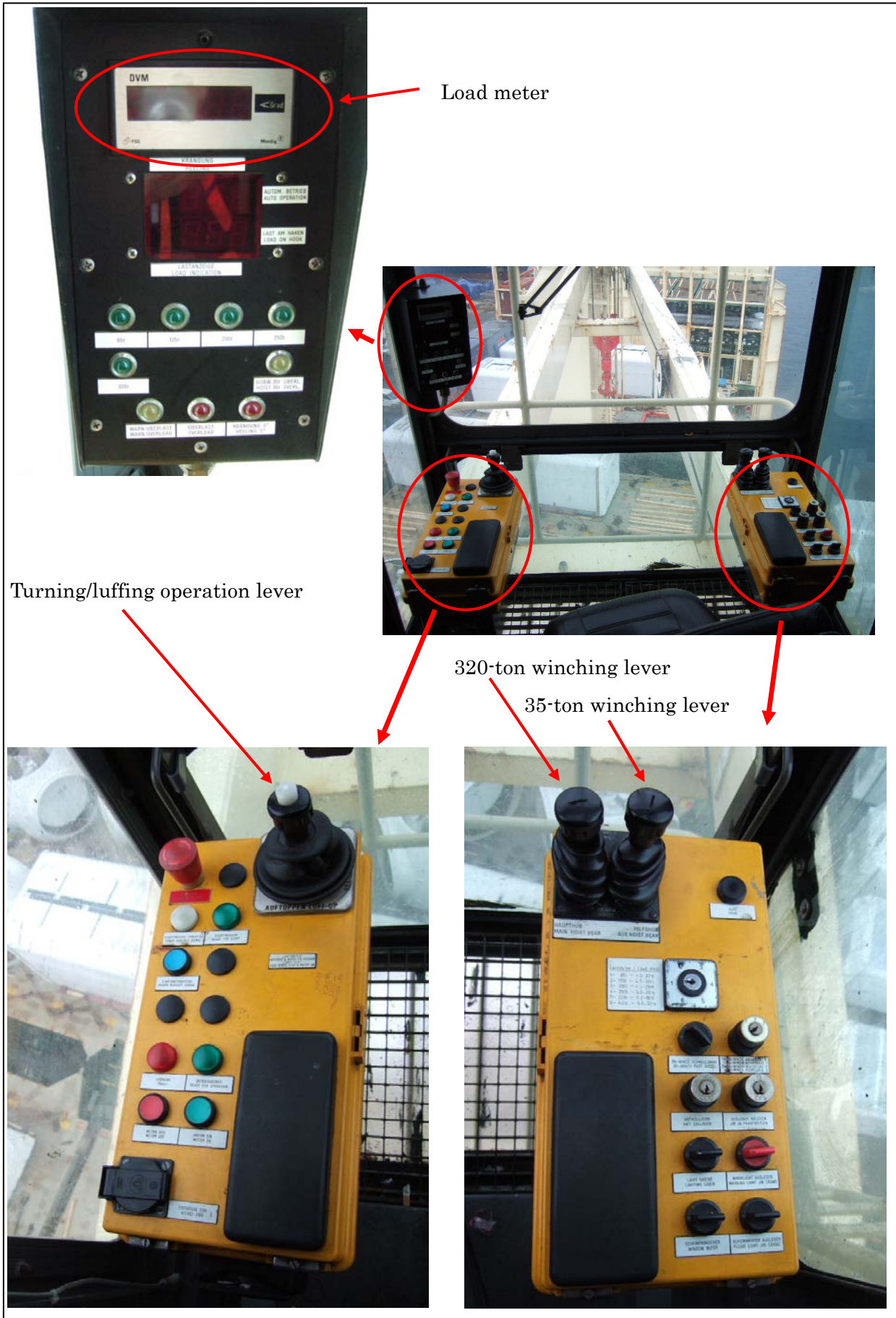
Picture 9—Operator's Cabin of Crane No.3
