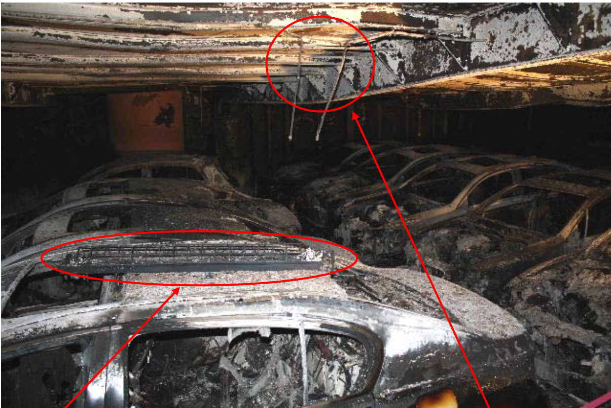
A fluorescent light was found to have fallen here
