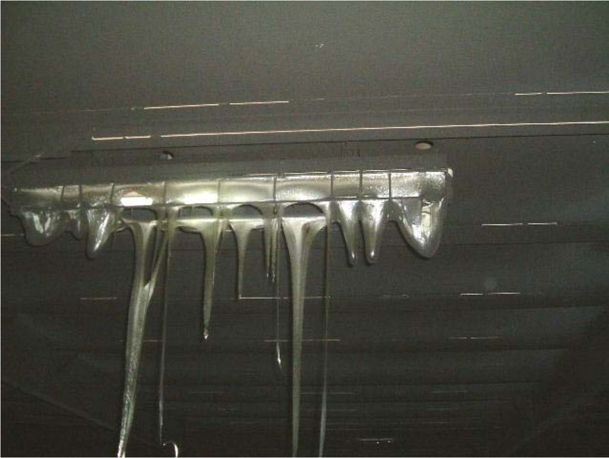
Photo 3: Fire Damage Situation of Fluorescent Lights
