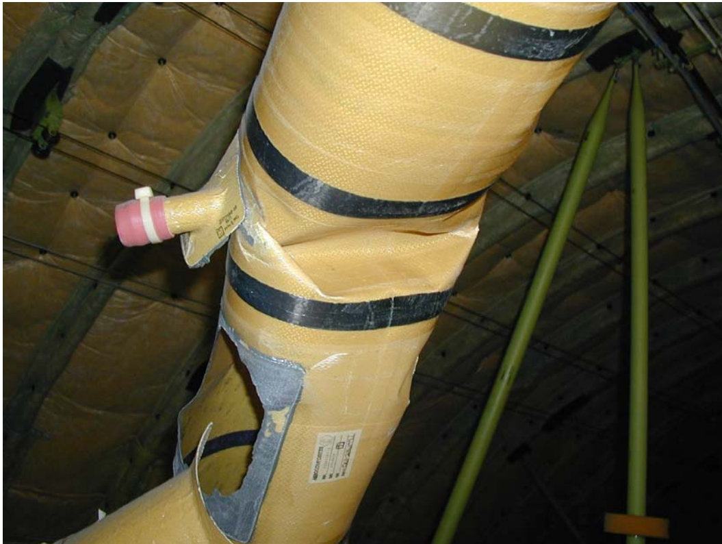
Photograph 3 Smash and Separation of Duct
