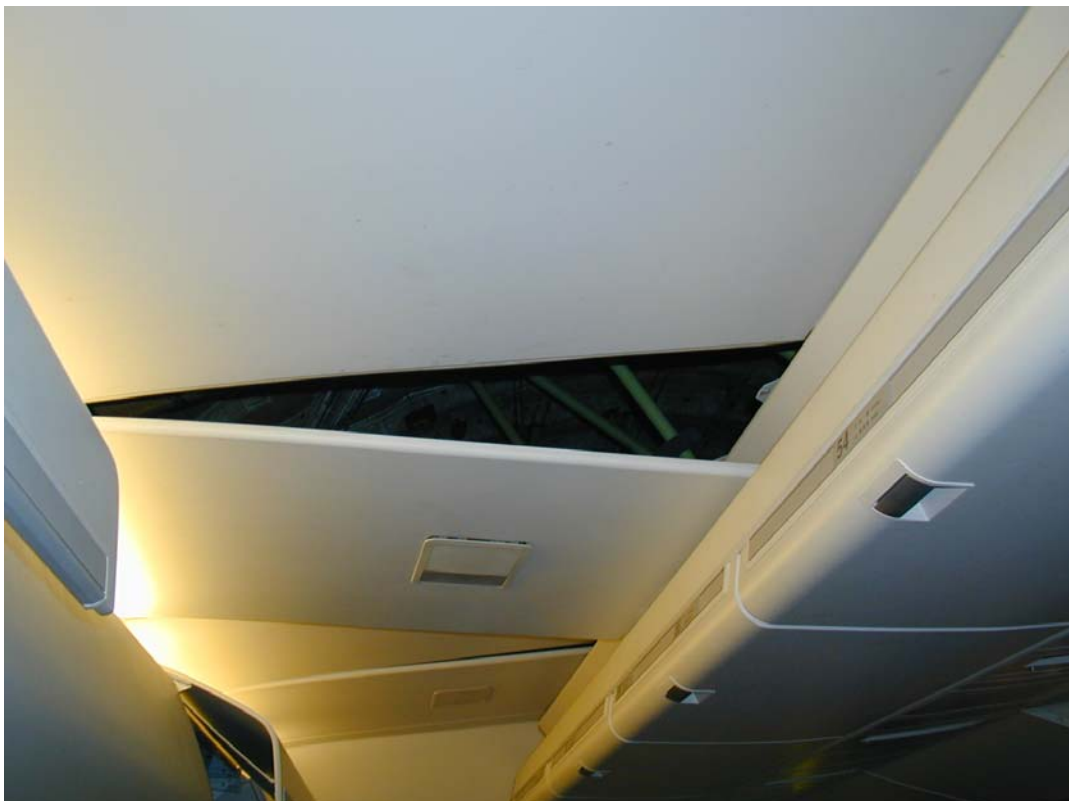
Photograph 2 Ceiling Panel out of place
