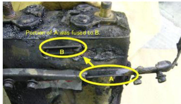
Fig. 2.11.5-2: Cell 6 and Brace Bar
