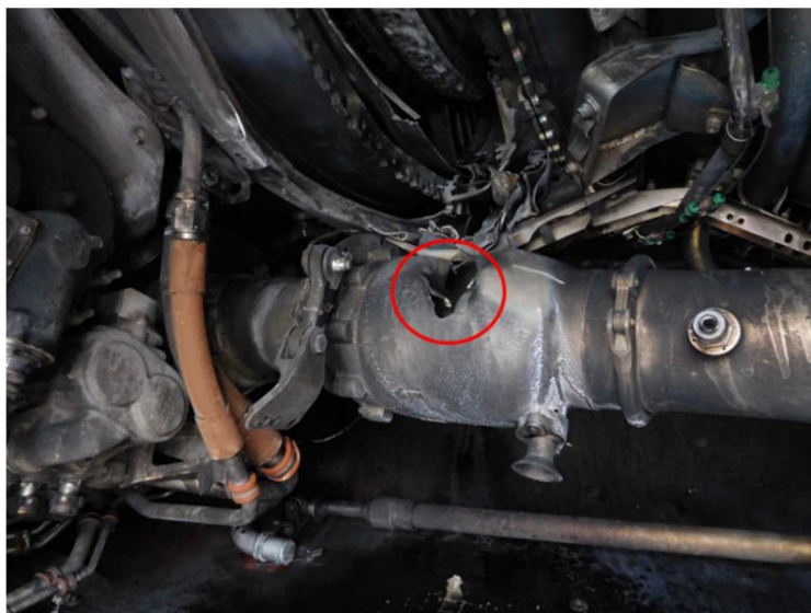
Photo #8. A Hole opened in Air Starter Valve
