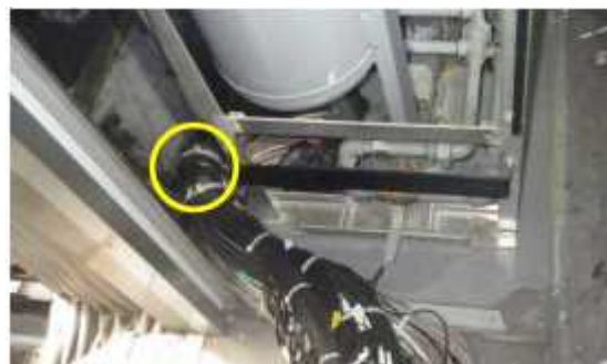
Wired status viewed from aisle side, broken in back side of the circled bundle of cables
