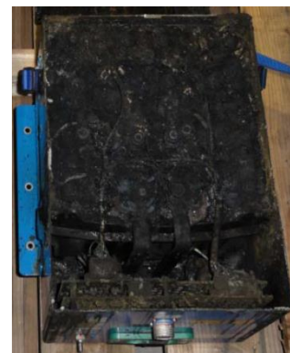
Interior of main battery
