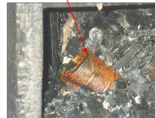
Ashtray Found under Stairway
